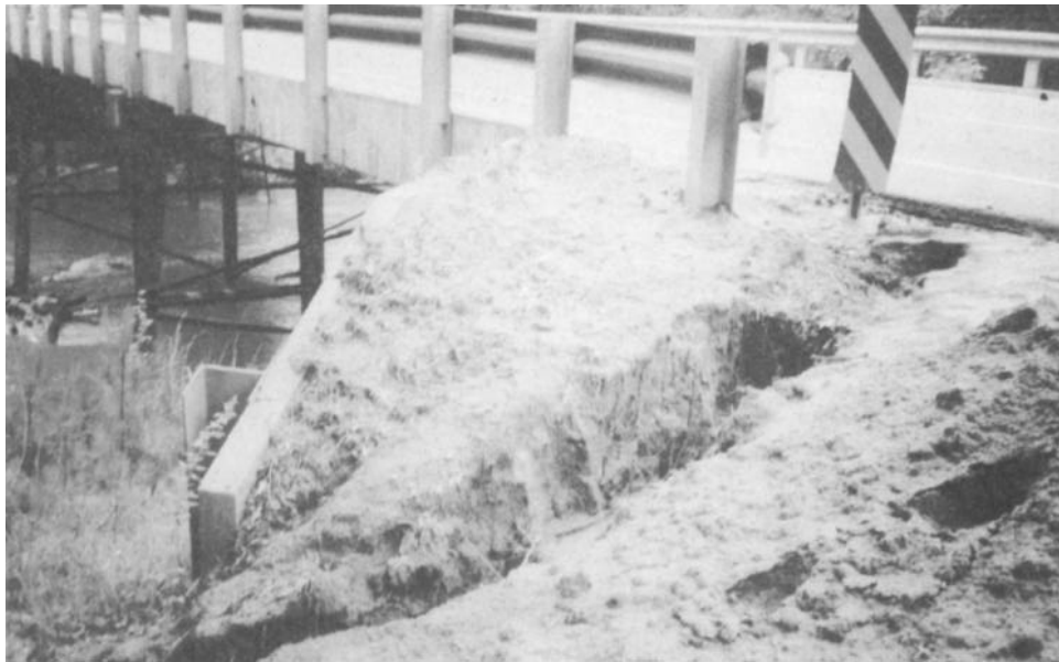
Figure 5-25. Embankment erosion due to improper drainage. (Sheet 1 of 2)
