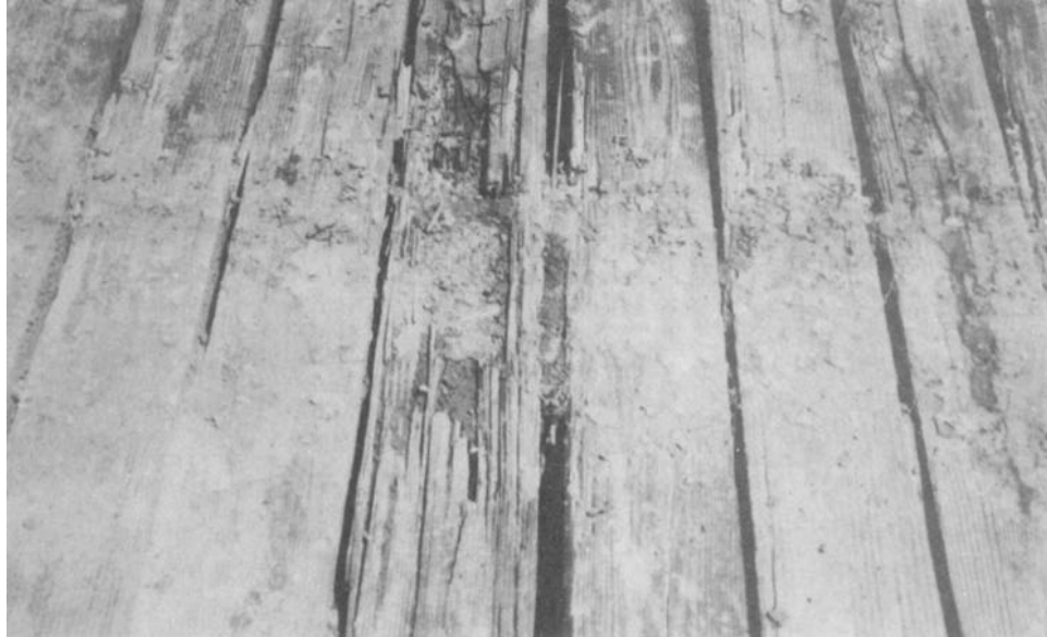
Figure 5-16. Slight and advanced wear on a timber deck (mechanical abrasion wear also present).
