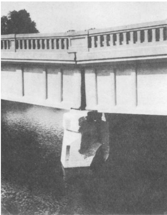
Figure 5-22. Movement due to scour.
